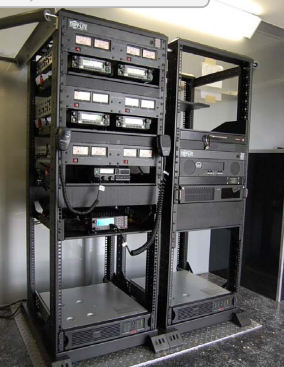
SyTech RIOS Rackmount Installation
