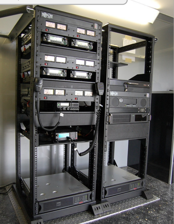
SyTech RIOS Rackmount Installation
